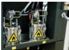
Best accessibility: flux storage tanks for the flux supply
